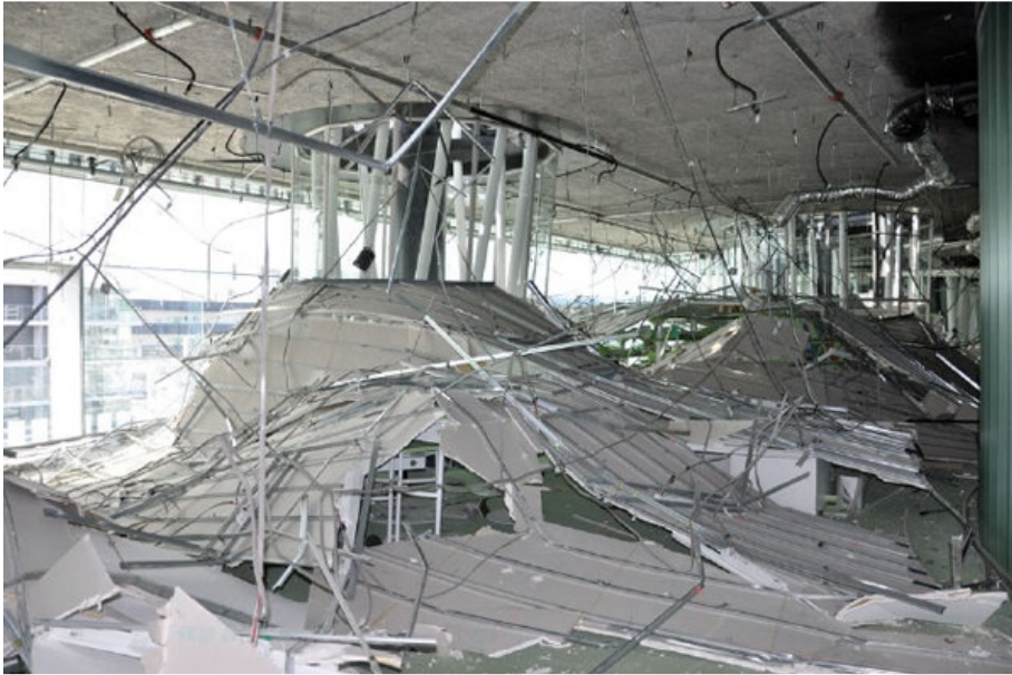
Non-structural damage: Japan earthquake March 2011
