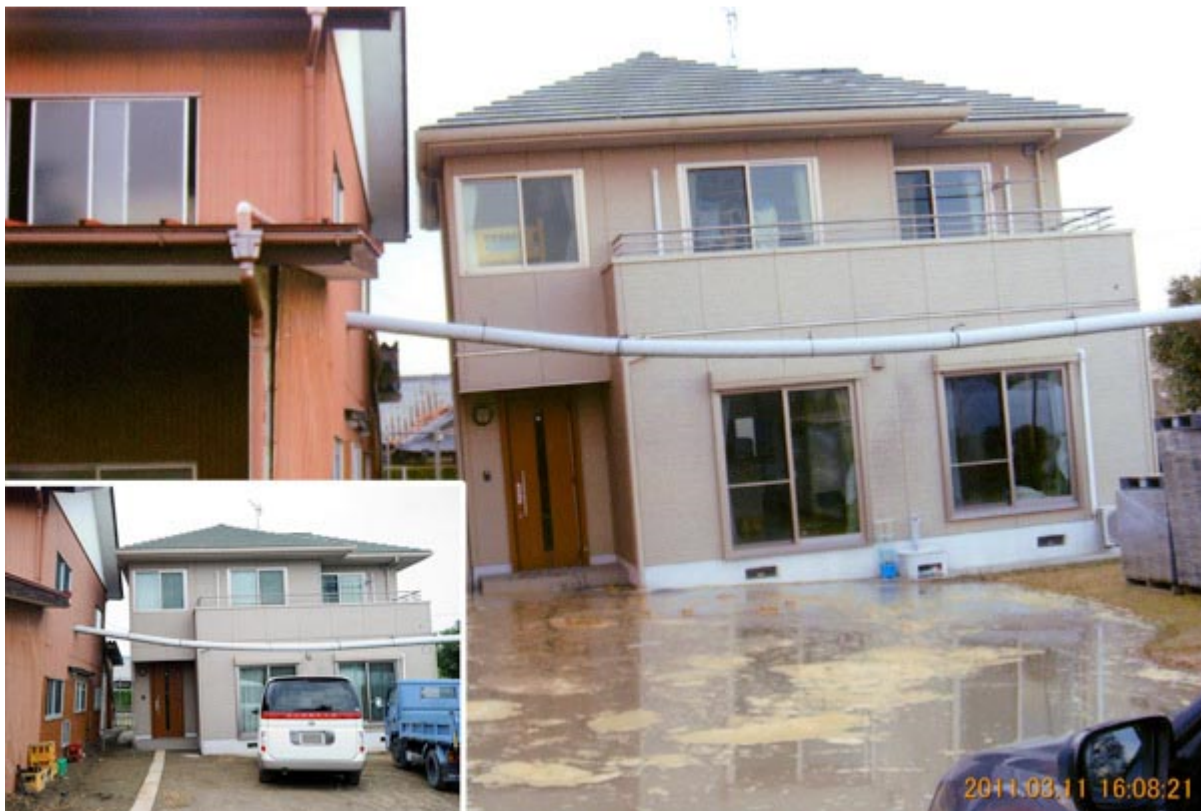
Liquefaction immediately following the Tohoku earthquake left this house with a permanent lean. Source: japanpropertycentral.com
